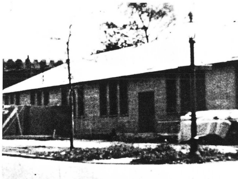
Fig. 21 New Chemistry Building under construction, October 1942. Facing southeast from corner of 56th Street (left) and Ingleside Avenue (right). (XBB 768-7461)
